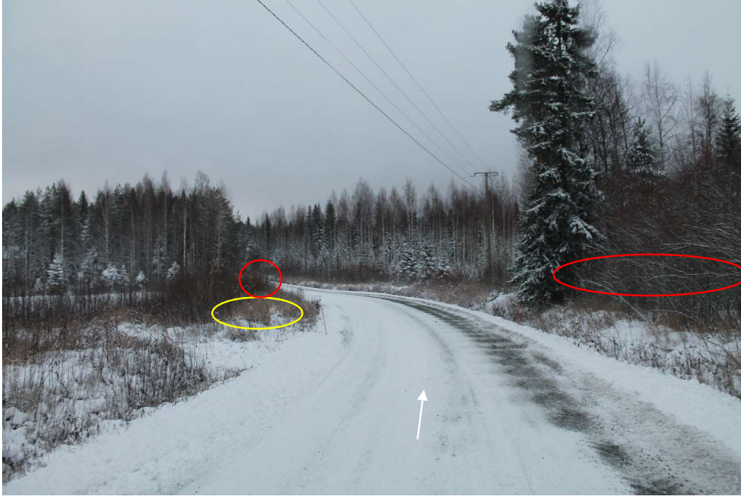
Pos 34/Pic 65. Road 16235 (Keskimmäisentie). Road need to be levelled. Marked trees need to cut. Oversail area need to be free in inner curve. Road need to be fixed according to specifications for site roads.
