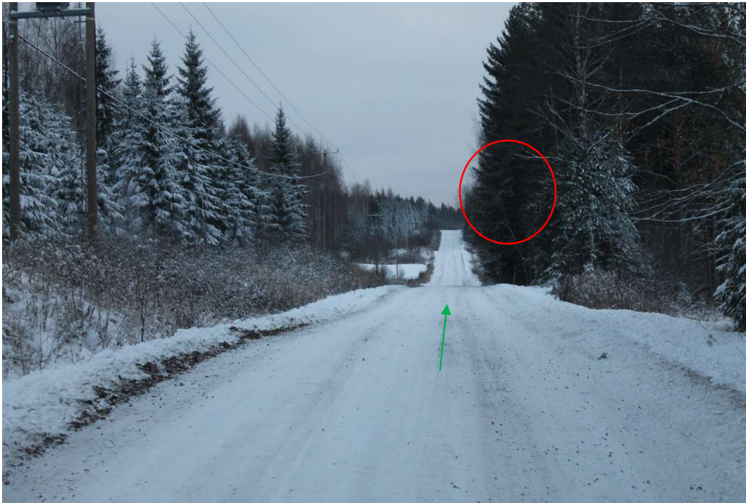
Pos 40/Pic 77. Road 16235 (Keskimmäisentie). Marked tree branches need to cut. Crest, road need to be levelled. Road need to be fixed according to specifications for site roads. Green arrow points driving direction for Entrance B.
