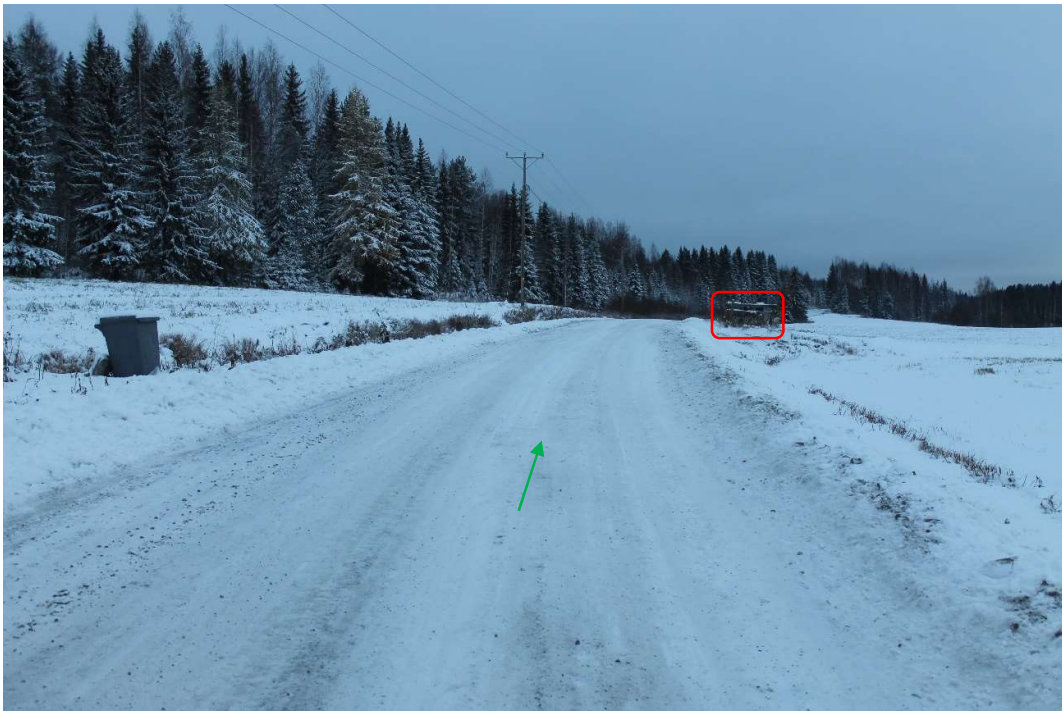
Pos 39/Pic 74. Road 16235 (Keskimmäisentie). Road need to be levelled. Road need to be fixed according to specifications for site roads. Marked mail box need to be removed. Green arrow points driving direction for Entrance B.
