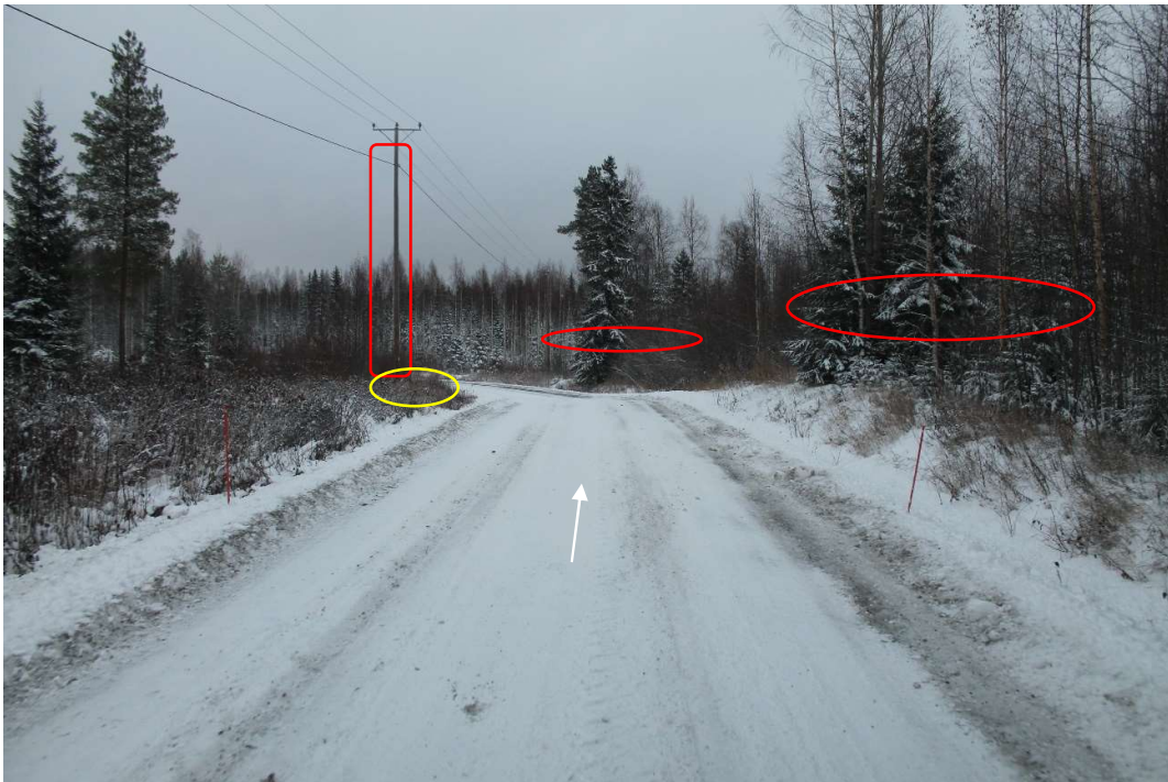
Pos 34/Pic 64. Road 16235 (Keskimmäisentie). Crest, road need to be levelled. Marked pole need to be removed. Marked trees need to cut. Oversail area need to be free in inner curve. Road need to be fixed according to specifications for site roads.
