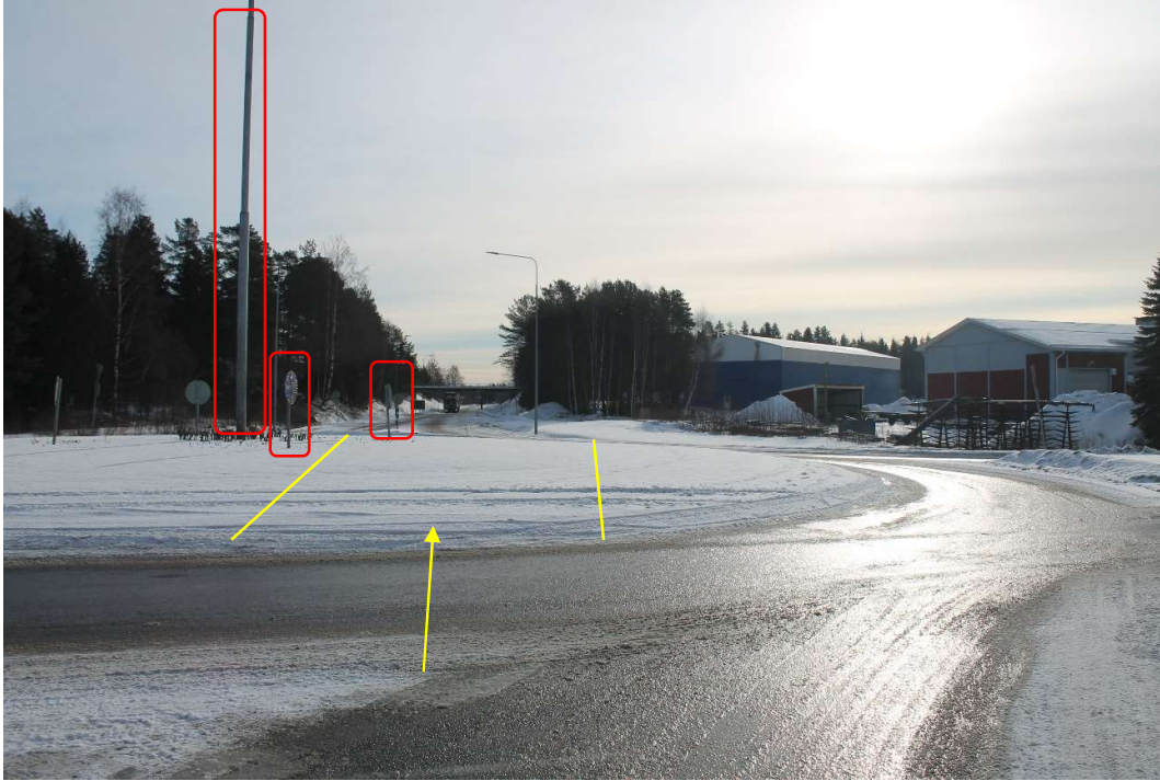
Pos 45/Pic 87. Roundabout Lapaluodontie. https://goo.gl/maps/fNoSyewtX85WBptj7 . Marked lamp post and signs need to be removed. Marked area need to be filled and drivable.
