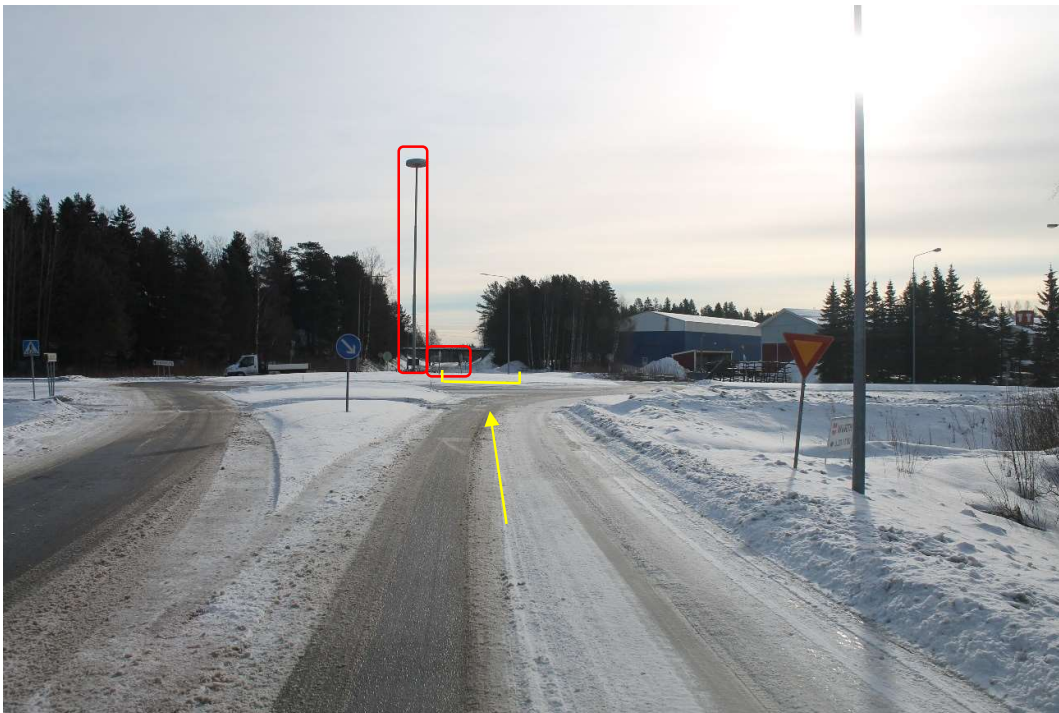
Pos 45/Pic 86. Roundabout Lapaluodontie. https://goo.gl/maps/fNoSyewtX85WBptj7 . Marked lamp post and signs to be removed. Marked area need to be filled and drivable.
