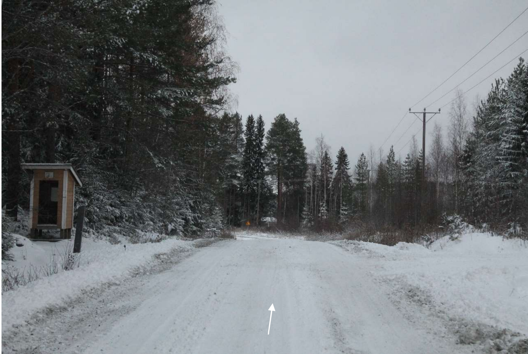
Pos 35/Pic 67. Road 16235 (Keskimmäisentie). Crest, road need to be levelled. Road need to be fixed according to specifications for site roads.
