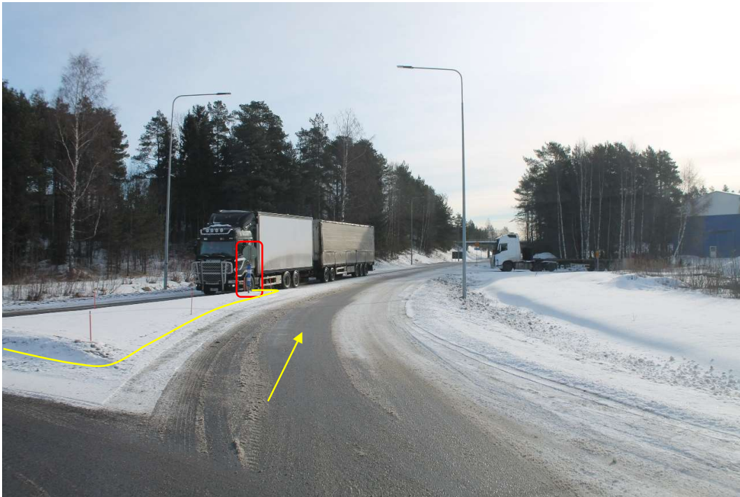
Pos 45/Pic 88. Roundabout Lapaluodontie. Marked sign need to be removed. Marked area need to be filled.
