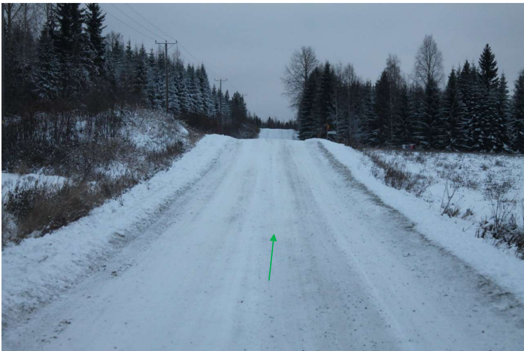
Pos 41/Pic 78. Road 16235 (Keskimmäisentie). https://maps.app.goo.gl/vq2kaHPwBVwbMojE8 Crest, road need to be levelled. Road need to be fixed according to specifications for site roads. Green arrow points driving direction for Entrance B.
